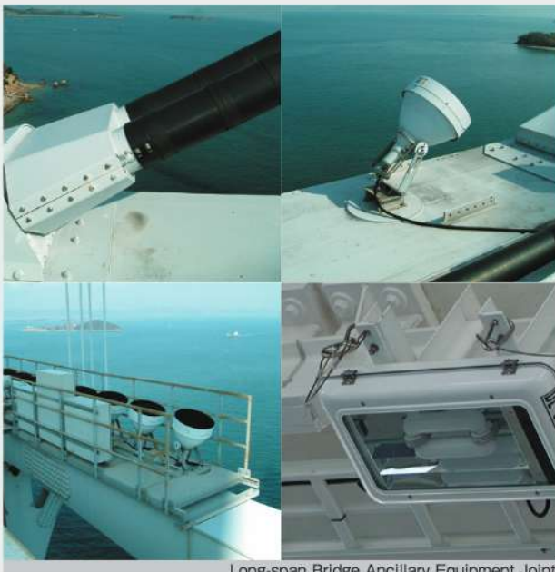
Long-span Bridge Ancillary Equipment Joint
