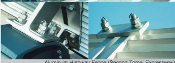
Aluminum Highway Fence (Second Tomei Expressway)
