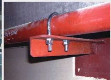
Piping in Power Plant
